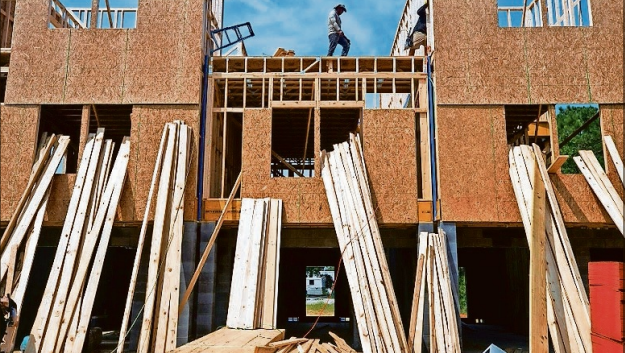
Construction workers walk across a townhome being built as a part of Bermuda Pointe Towns.
